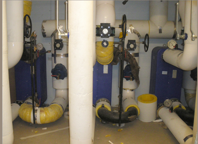
Energy Transfer Station (ETS) at The City of Calgary Municipal Complex (pictured above). The ETS has a significantly reduced space requirement when compared with conventional boiler rooms.
